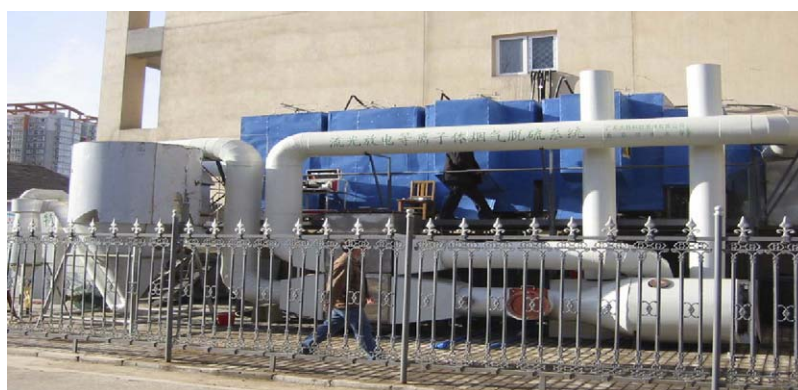
Fig. 2. Outward appearance of the 12,000 \text{Nm}^3/\text{h} streamer plasma flue gas desulfurization system.
